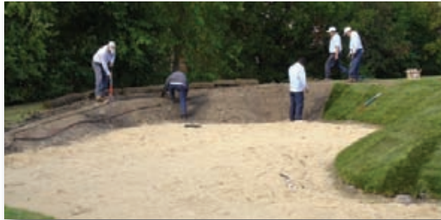
Installing drip irrigation while re-sodding the bunker face at the same time.
