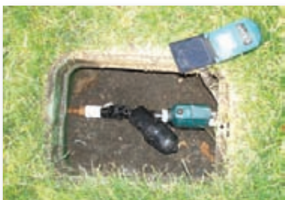
Tying the drip line into existing irrigation with control components was easy to do.
