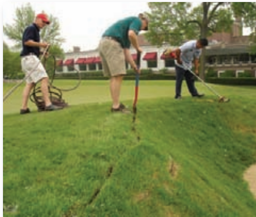
The crew at Park Ridge Country Club cuts a trench for the new drip tubing.
