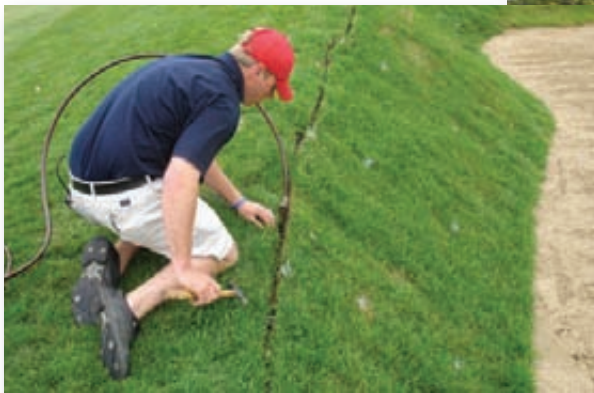
Just tap it in... Sod staples are used to hold the drip line at the bottom of the slit trench.
