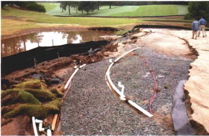
Covers can only do so much against a heavy rain on this green. This picture shows the uncontrollable aspects of a renovation that weather created – washing away and exposing irrigation pipes and gravel layers.
