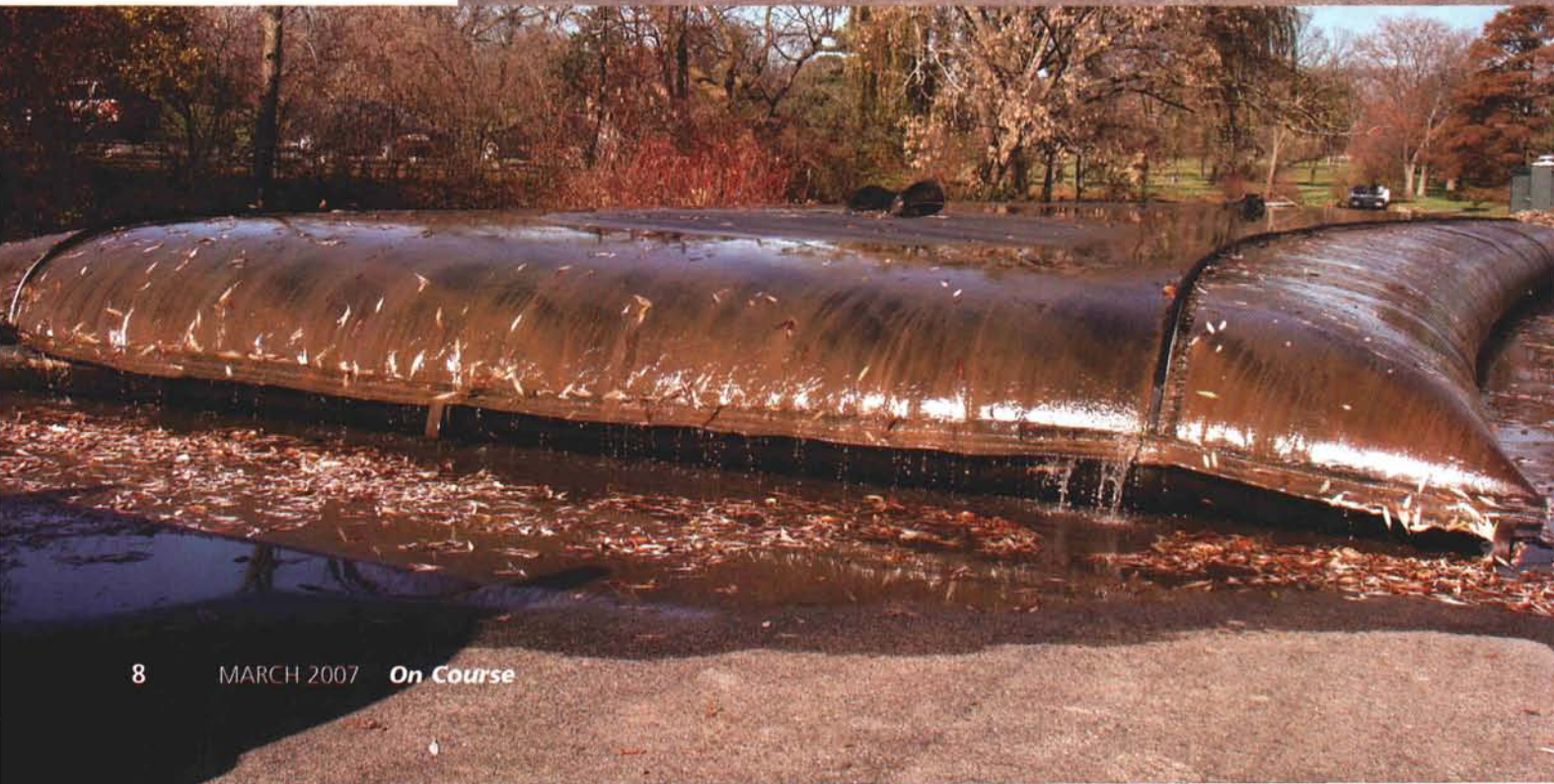
Below: The silt bag at the end of a day of sucking up sediment. It would fill to four feet high upon completion of the divers shift and water would drain throughout the night leaving only sediment in the bag.
