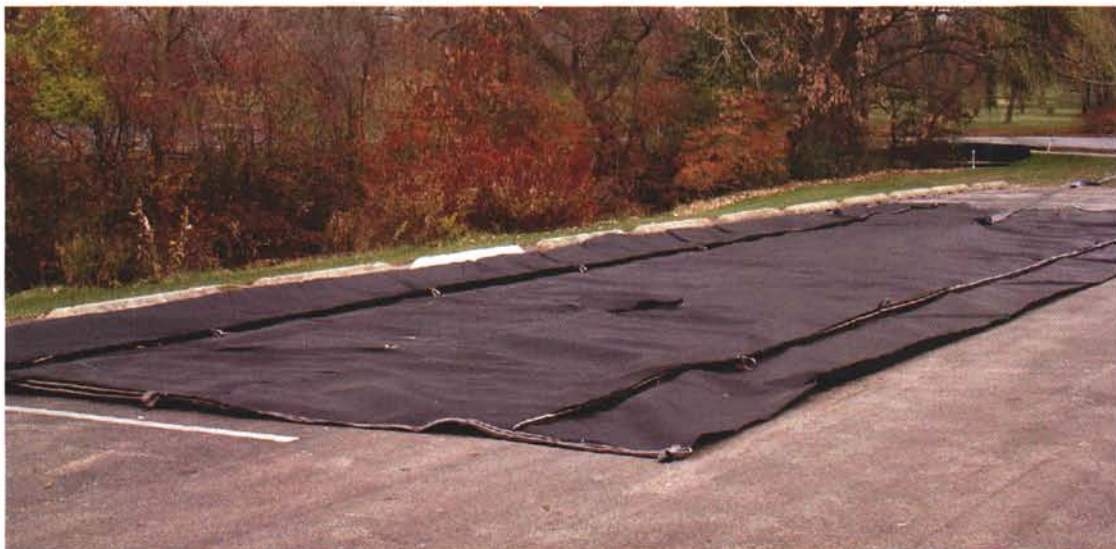
Right: The 74' x 45' silt bag prior to filling sits on a seldom used parking lot adjacent to a creek.
