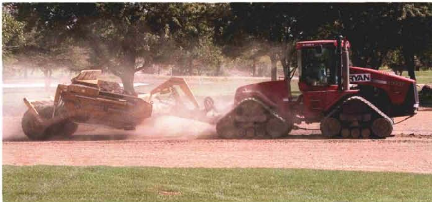
Let the construction begin as the superintendent acts as the representative of the owner overseeing what will eventually become his or hers to manage.
