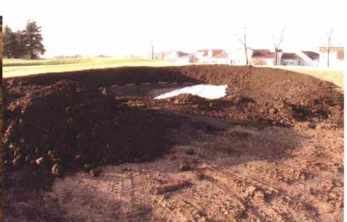
Changing the shape of the bunkering around the 8th Green on the Blue Course.
