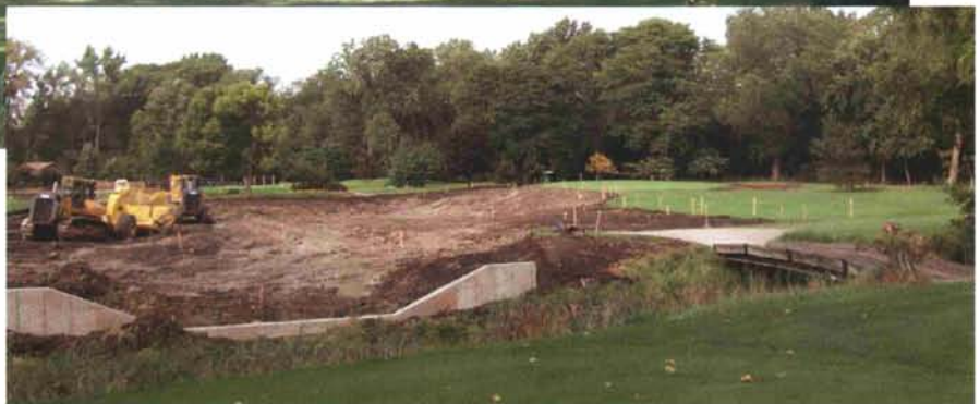
5th hole as construction begins and cottonwoods are absent. Pond excavation and weir structure are underway.
