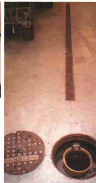
Catch-basin in floor with filter screen. The whole floor drains to a 20-foot trough that runs to the catch-basin.
