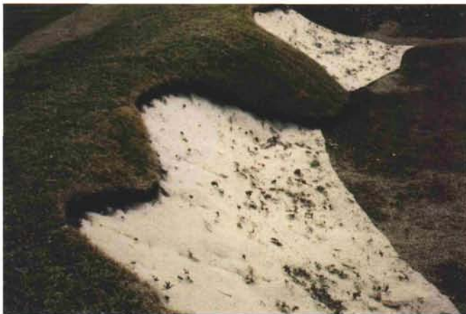
Sand Trapper bunker matting was installed along all bunker faces during construction.
