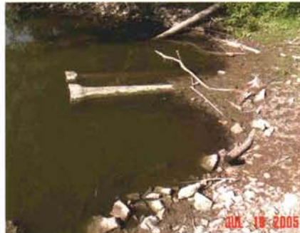
The 6", diesel-powered pump Fox Valley Country Club uses to draw irrigation water from the Fox River.
