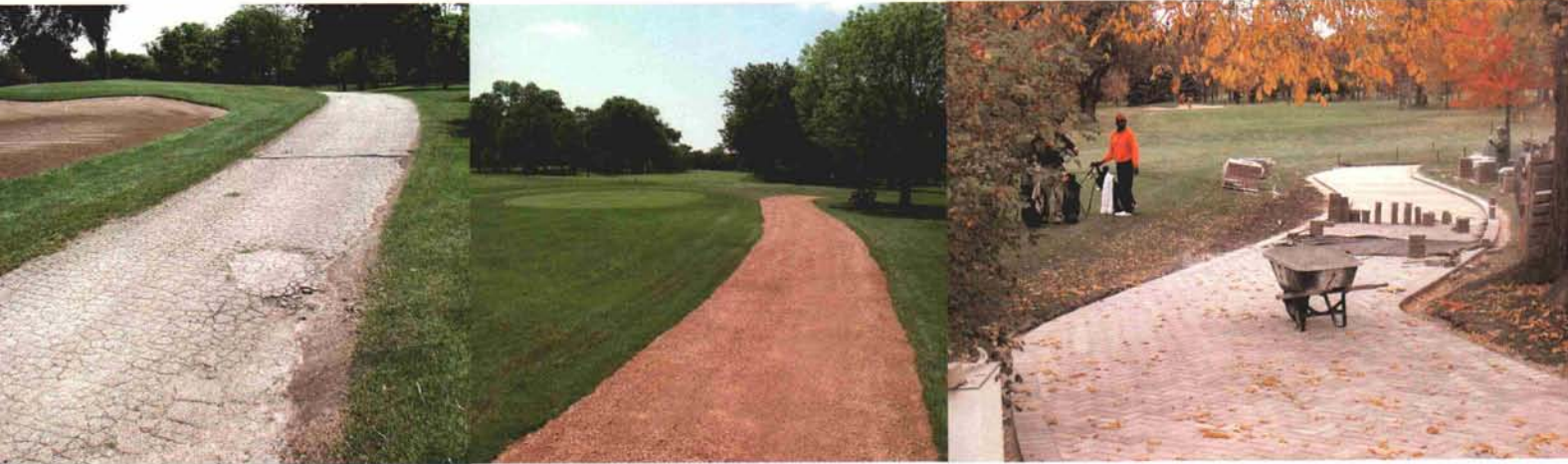
Renovation saw removal of all asphalt cart paths and replacement with stone paths in most cases. Where traffic is too heavy for granite gravel paths, rustic paving brick was installed, as on no. 10.
