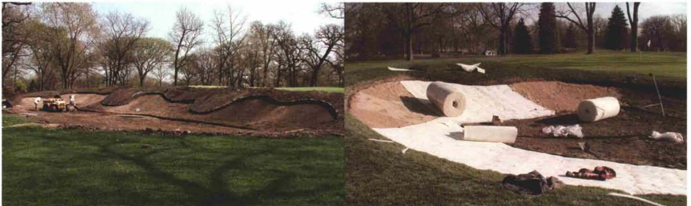
(Left) After old bunker sand was removed, as much as three feet-plus deep, the original bunker configuration became apparent. These contours were used as a guide to form the new bunkers as we built the edges by hand. (Right) Bunker construction in progress.
