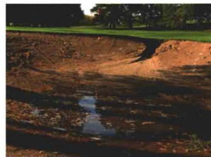
Surface runoff into a bunker and poor internal drainage are evident by washed-out sand and "the pond."
