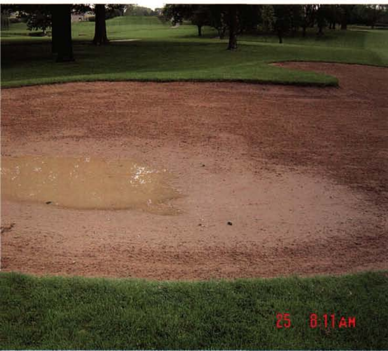
A sand bunker that has inadequate drainage. Notice the different colors of sand from years of contamination.
