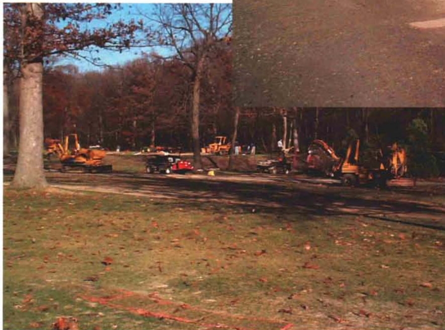
The changes requested by the USGA were extensive enough to warrant replacing the "maxed out" 1978 hydraulic irrigation system at the same time as the rest of the construction work. Here, irrigation installation.
