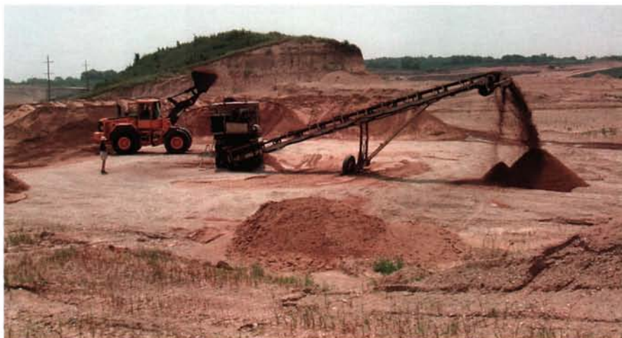
Inspecting the blending site for a hard surface during prequalifying visits to local sand suppliers is necessary to prevent contamination of the root-zone stockpiles once produced.
