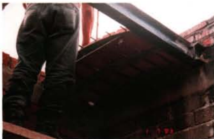
Mason building the roof/ceiling, using bricks in an arch form. Notice bow-type braces to support the bricks while the mortar dries.
