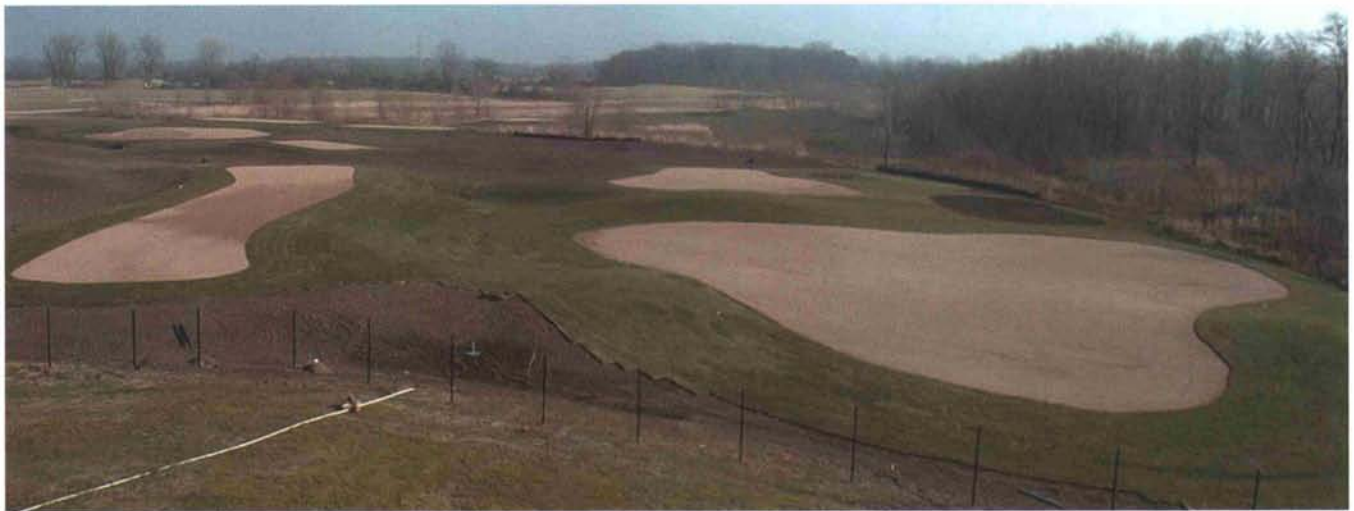
Thanks to a mild fall, construction on the three-hole short course at Midwest Golf House was proceeding nicely as of late November, 2001. (See more photos at www.cdga.org .)
