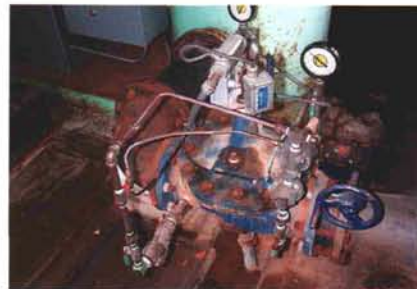
Inside CGC's old pump station.
