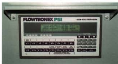
Data control pad for pump station.
