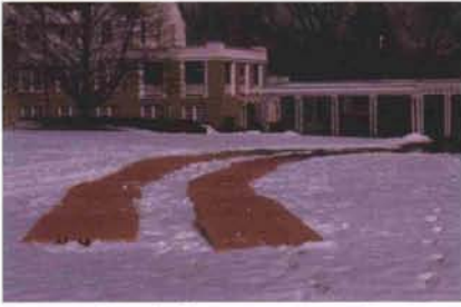
Plywood path for cement trucks to traverse to minimize golf course damage.
