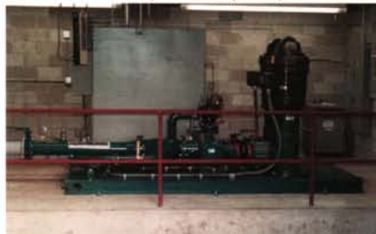
Inside of new pump station at CGC.
