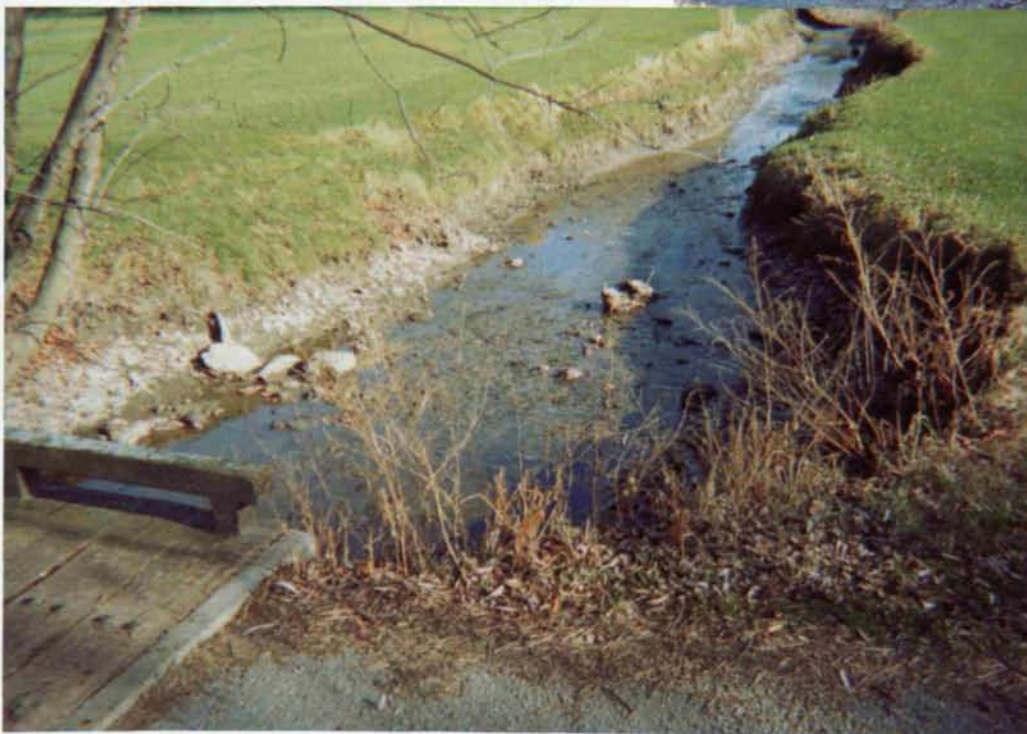
Eroded creek bank caused by restricted flow upstream.
