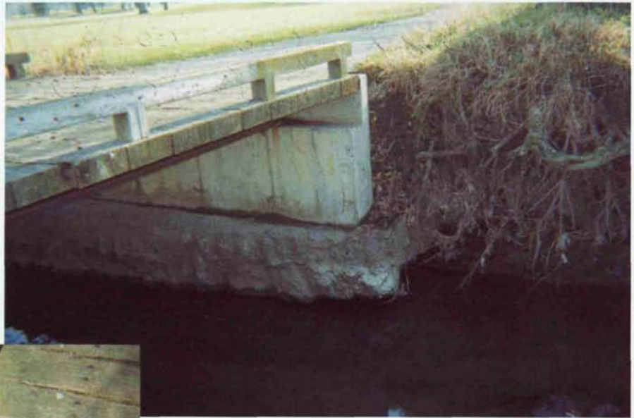
Eroded bridge foundation. Note exposed roots of adjacent tree.
