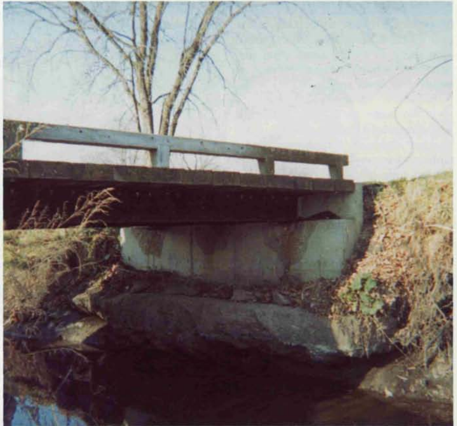
Exposed bridge footing —spalled concrete is caused by the foundation settling.
