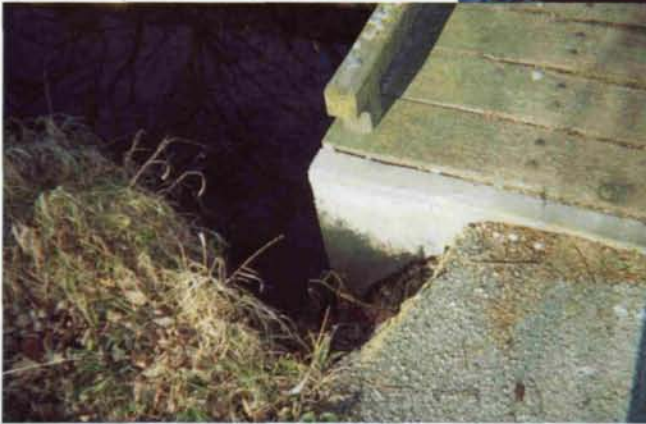
Cart path erosion.
