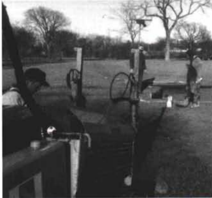
To eliminate surface disruption, drain lines can be put in with horizontal boring equipment.
