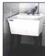
Wash tub with emergency eye-wash
