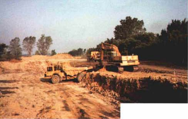
9/8/91—During lake excavation, track-hoe excavates subsoils while articulating dump trucks haul the cuts to the fill sites.
