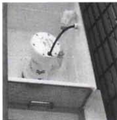
Computerized pump system keeps fluids within 1/4 inch depth, stainless steel removable screens filter large debris.
