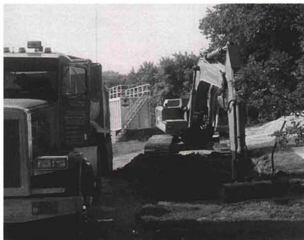
Redigging hole in cleanup of contamination. Portable water tank in background for excess water.
