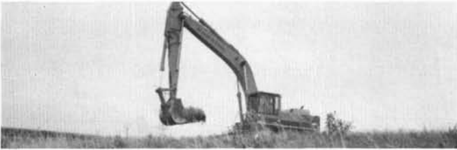
Large backhoe scraping up the prairie to be moved to a new site.
