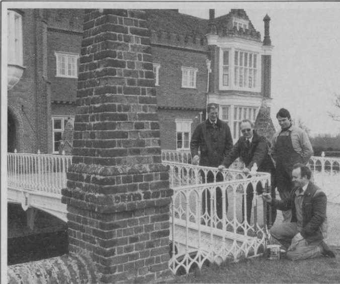
Giving the final touch to one of the new railing sections for the 180-year-old Ransomes bridge is Mr Keith Gardiner the estate carpenter. Looking on, (left to right) are: Lord Tollemache: Ransomes Foundry Manager, Mr David Wright and Mr Paul Winbolt a local garden furniture specialist.
