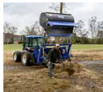
MAIN ABOVE: Ground cleared and surface prepared ready for heather brashings. INSET ABOVE: Spreading heather brashings over prepared area
