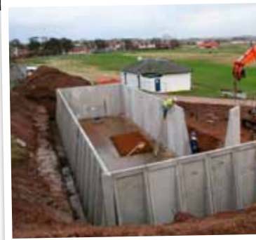
The initial cost of a reservoir can be recouped over a period of time and they provide an additional protective measure against drought orders Courtesy of MJ Abbott Limited
