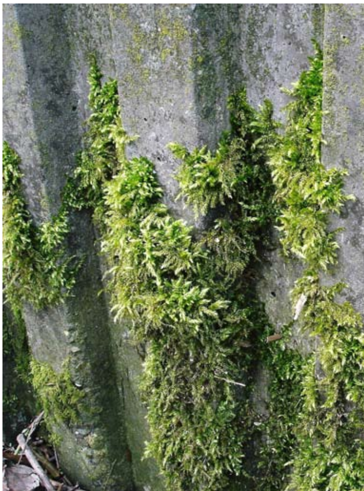
Moss will readily grow on a wide range of vertical as well as horizontal surfaces
