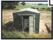
Irrigation Pump Housing
