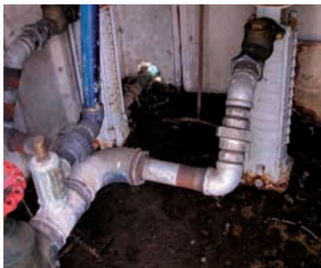
A wet pumphouse floor needs addressing
