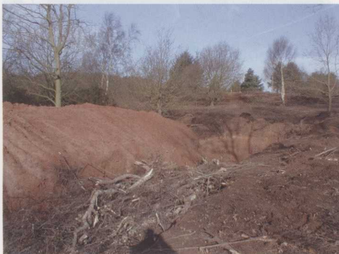
Creation of one of five giant hibernacula (hibernation chambers) in land cleared of trees at Notts Golf Club. These are constructed by burying sections of cut trees and brushings with one end being left open at the south side of the mound
