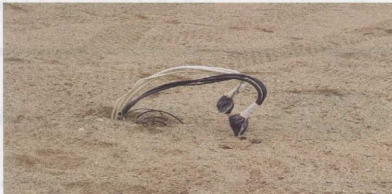
An example of good wire splices made using waterproof splice kits. Now they need to be placed in a valve box for protection and so they can be easily located later for troubleshooting if necessary
