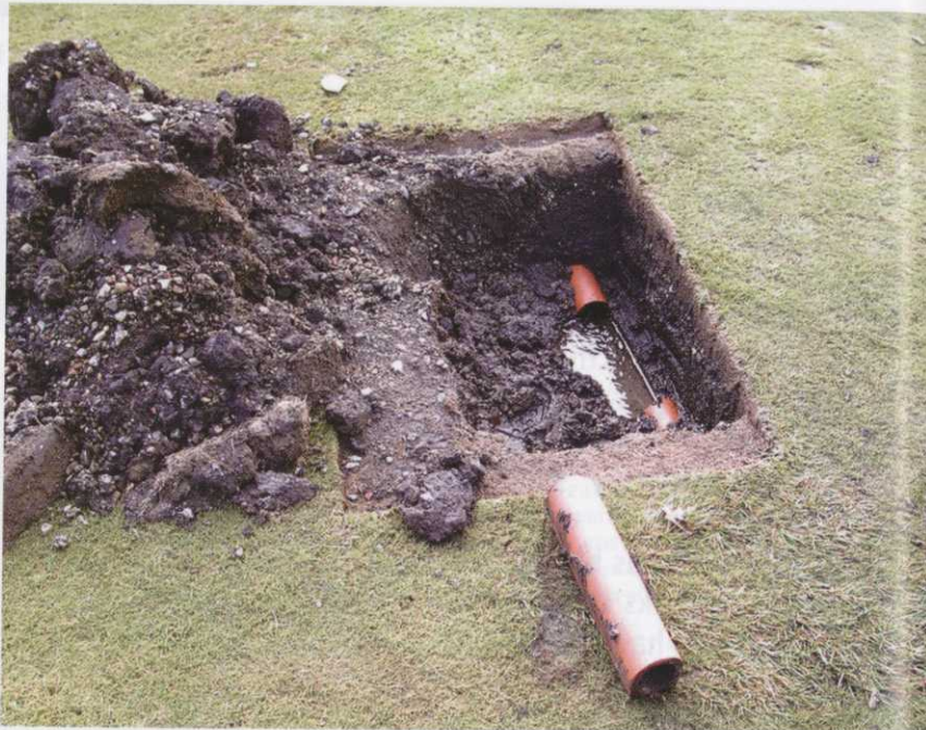
▲ Old fairway drains may need replacing with more appropriate and effective modern drainage systems.
