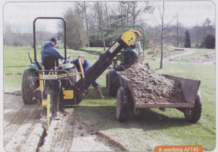
A working AFT45
