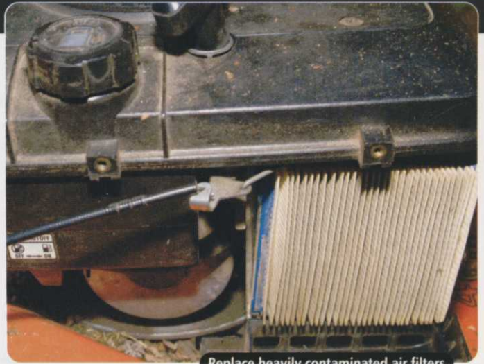
Replace heavily contaminated air filters
