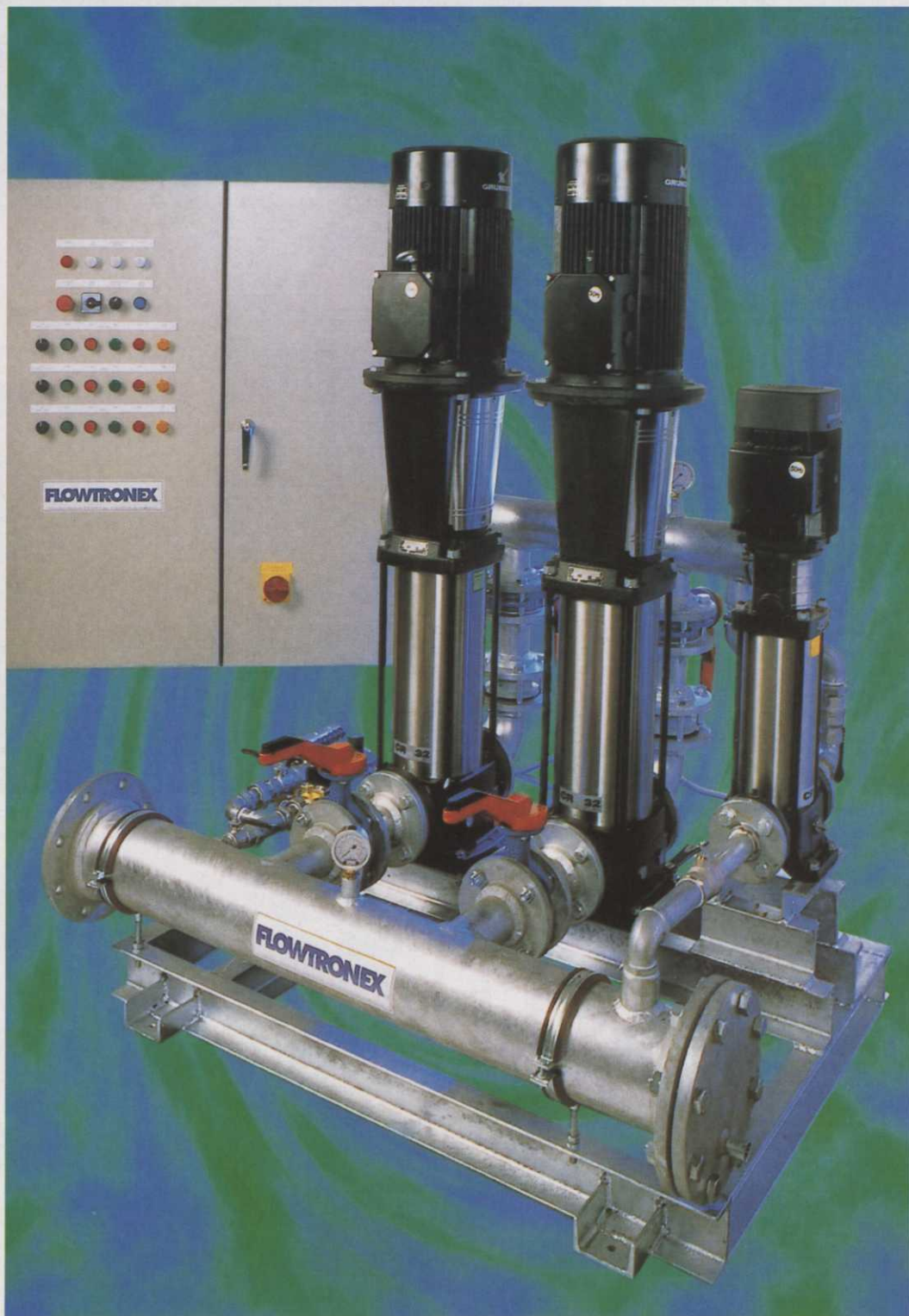
Variable speed pumpset installed at the Millennium Dome in London for landscape irrigation
