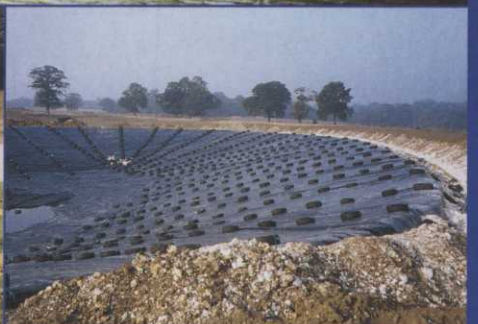
Eyhurst Golf Club: Reservoir Liner (exposed)
