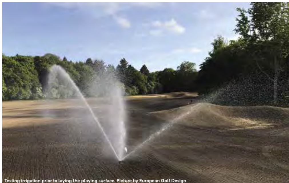
Testing irrigation prior to laying the playing surface. Picture by European Golf Design
