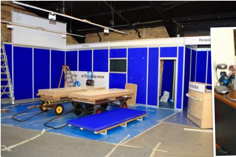
ABOVE: The BIGGA stand under construction, beside Tracey Maddison, working at BIGGA HOUSE
