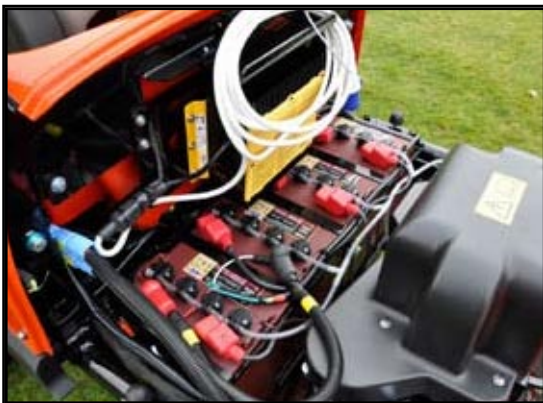
The battery charger is an integral part of the Eclipse 322, as is a centralised electrolyte top-up system. Although lithium-ion and other battery types grab the headlines, modern control systems and intelligent chargers ensure there is still a lot of life left in lead-acid battery technology.
