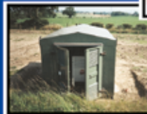
Irrigation Pump Housing
