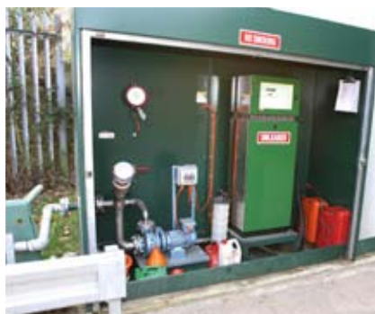
Storage of petrol is covered by a completely different set of regulations than diesel. Anyone looking into petrol storage needs to take specialist advice.
