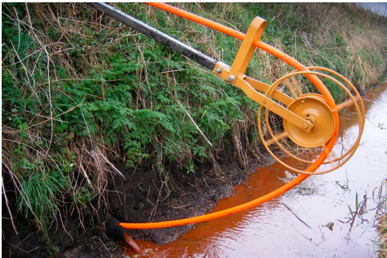
Ochre is a particularly common sediment found in primary drainage systems in certain parts of the country; note the rusty brown deposits flushed from the pipe pictured. Mastenbroek jettors are typically used for agricultural field drains, but there is no reason why they cannot be employed in sports turf drainage.
