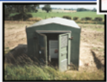
Irrigation Pump Housing
