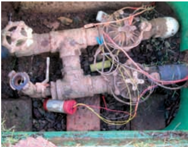
Poorly configured assembly with poor cable joints.
