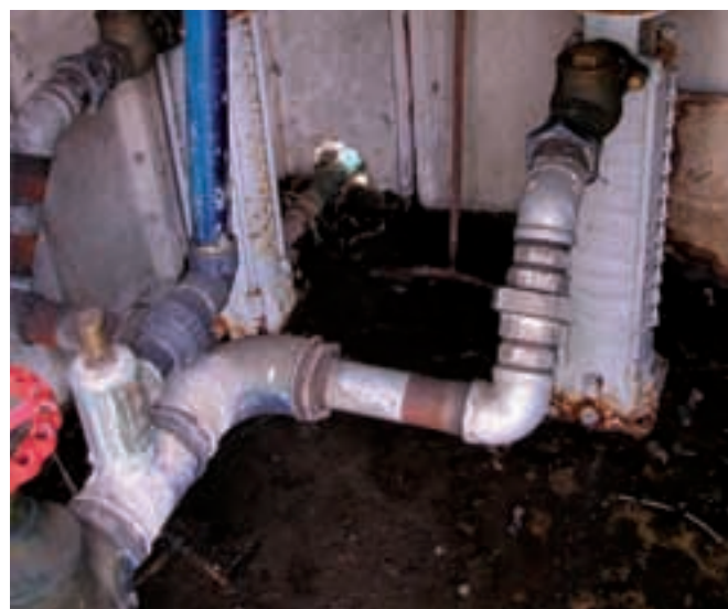
A wet pumphouse floor needs addressing
