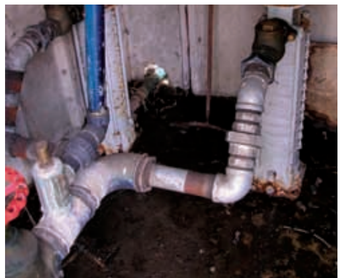
A wet pumphouse floor needs addressing
