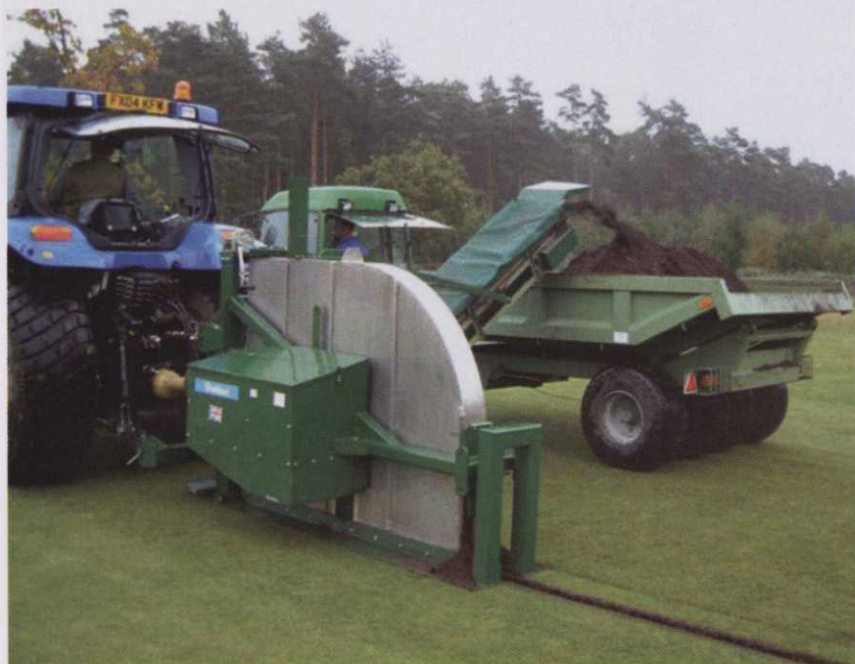
A Supertrrencher installing a 80mm diameter piped drain. There need be no disruption. The trailer has to spread the weight and the 4 wheels in line protect the turf
