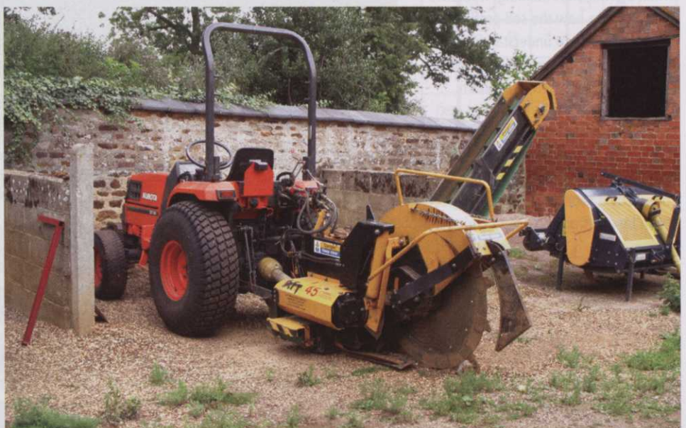
Ian Marshall, Head Greenkeeper at Wellingborough Golf Club, has carried out in house drainage and irrigation pipe installation on the course at Harrowden Hall using an AF Trencher, AF45, fitted with a Slitting Wheel. A job quoted out at £50,000 was carried out using the pictured combination for around £15,000.
