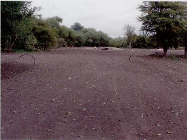
The new area was prone to flooding so the fairways were raised
