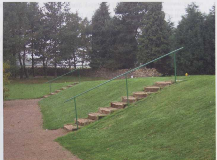
John sourced the materials and David did the installation of these stairs
