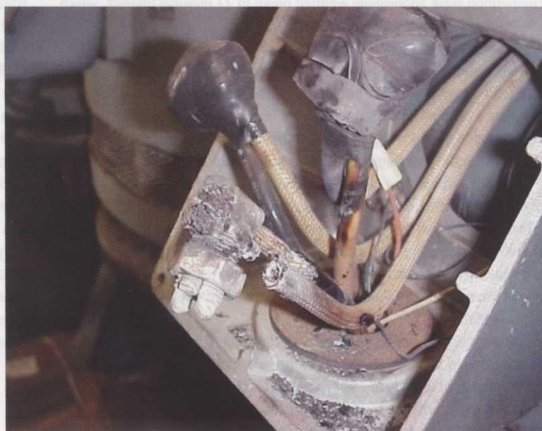
A loose wire connection can lead to failure, a safety hazard or expensive fire damage if not repaired. This one caused the failure and destruction of a pump motor, a very serious issue
