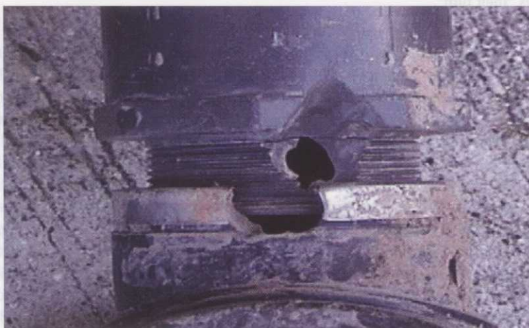
An example of how a small leak left untreated can turn into a larger problem later. Now the fitting, pipe and valve must all be replaced
